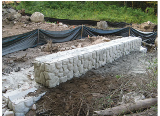
Figure 3. At grade, the abutments transition from plain rectangular blocks to blocks with a precast faux-stone face. Note the silt fences in the background.
